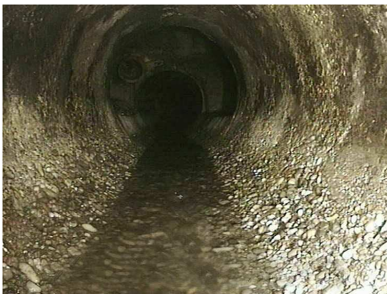
Figure: Examples of corrosion induced by the chemical quality of the wastewater
