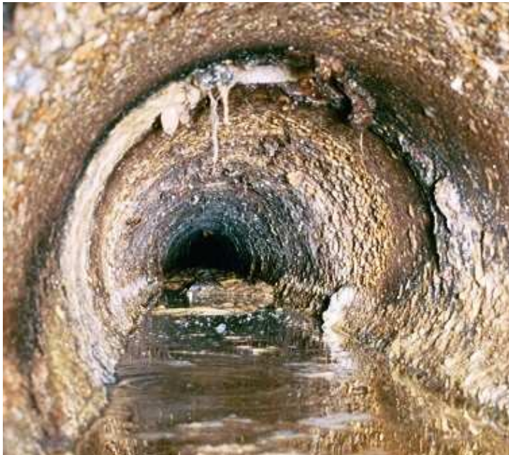
Figure: Corroded concrete pipe
