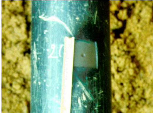
Photo 3: corrosion (diameter 5 mm, depth 0,5 mm)
