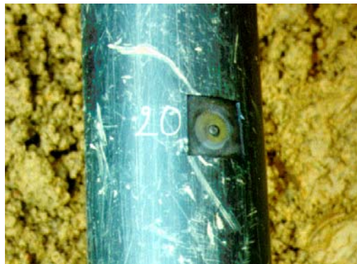
Photo 2: oxide (40x40 mm) and corrosion product
