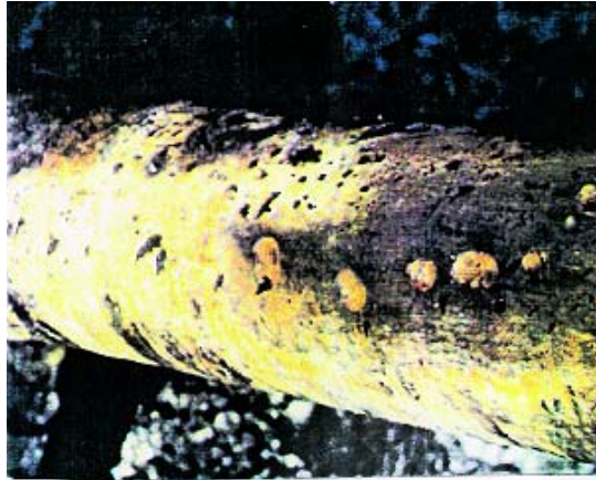
Figure 2- Typical a.c. corrosion on a bituminous coated pipeline (Reference 5)
