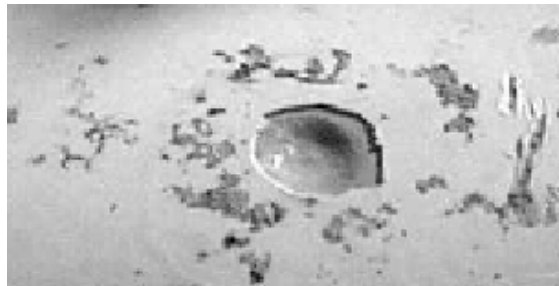
Figure 3 - Typical a.c. corrosion on an FBE coated pipeline (Reference 7)
