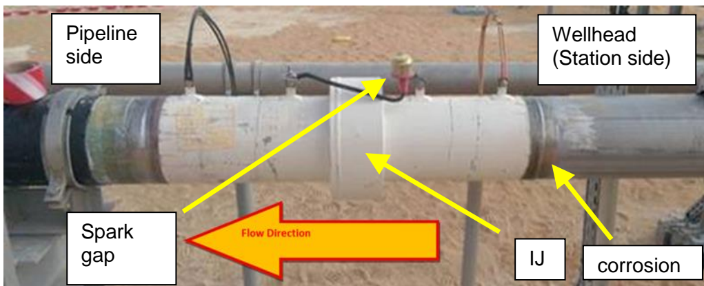
Figure 6. Failure at export line
