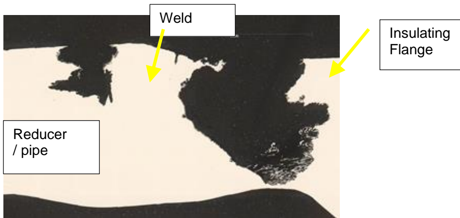
Figure 8 Cross section through a corroded weld area
