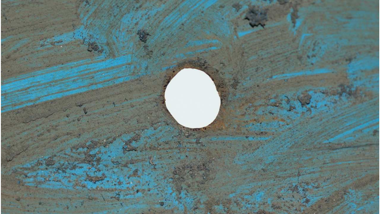
Internal view of corrosion perforation.
