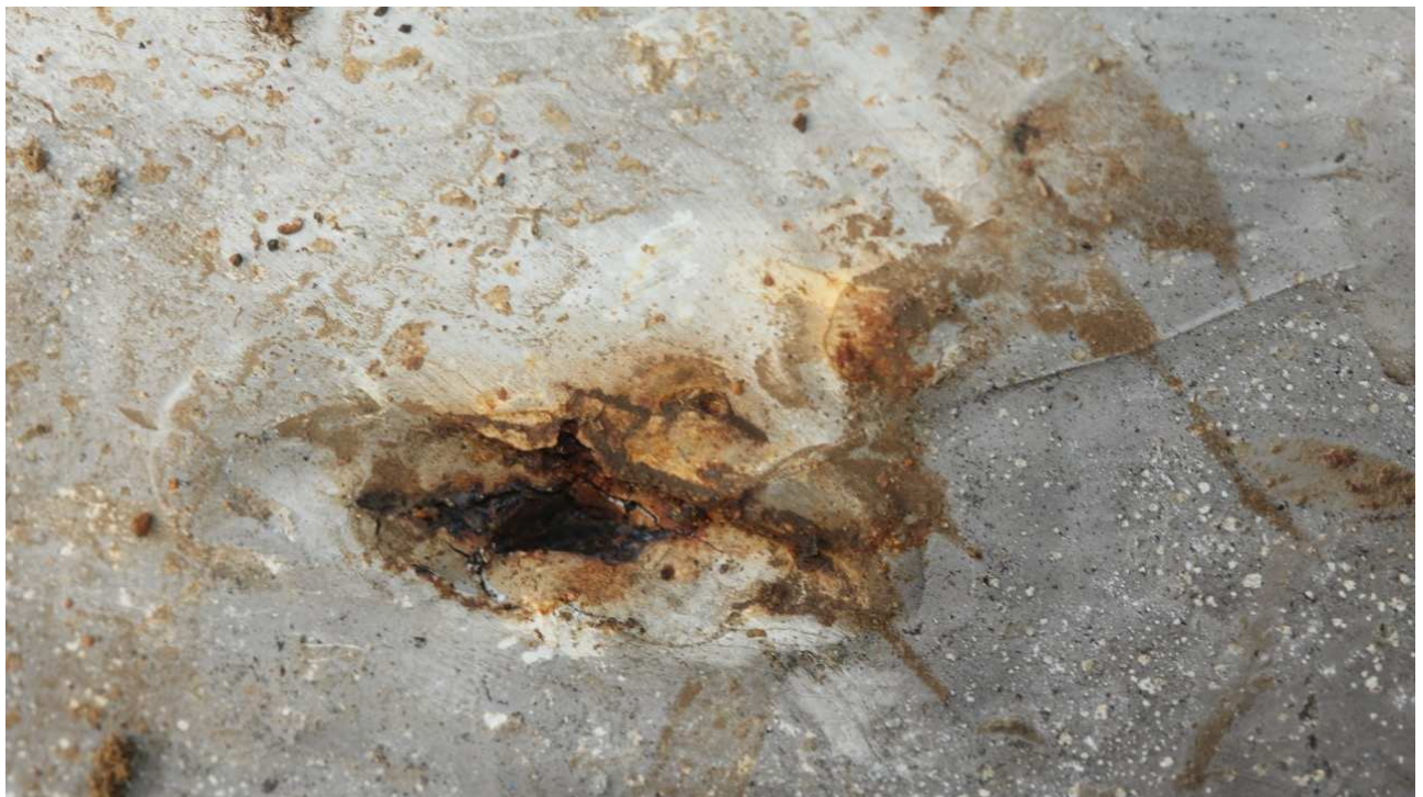
Corrosion site at location of coating damage prior to examination.
