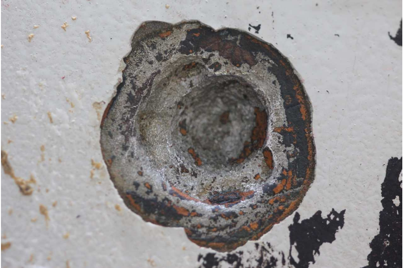
Corrosion pits showing shiny scalloped surface after removal of corrosion product
