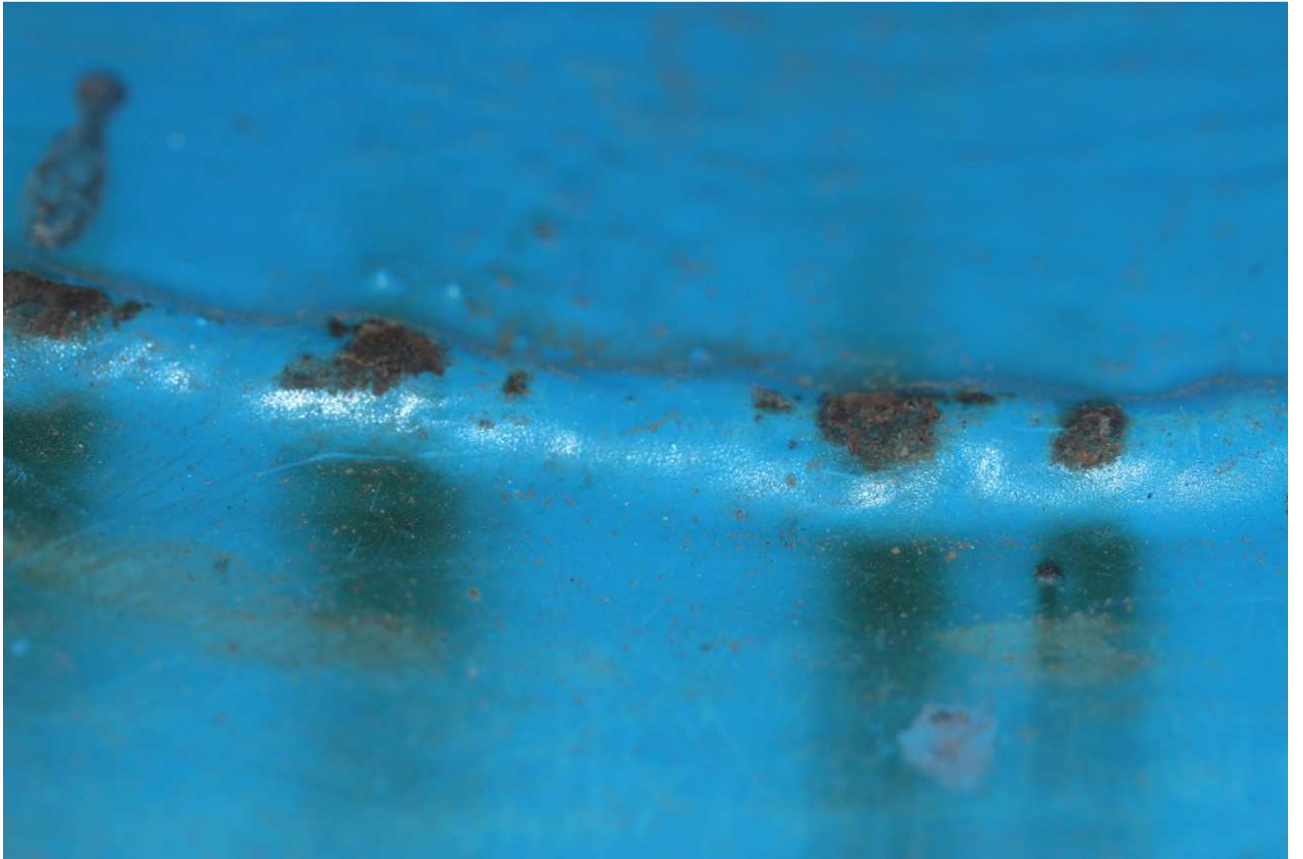
Internal corrosion at defects on internal weld - not significant.
