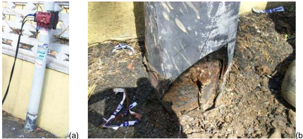
Figure 10. Application of guided waves on a lamppost (a) and corrosion defect localization (b)
