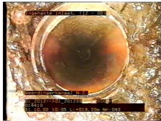
Figure 15: NL BBF (Infiltration) S&P: BAH (Defective connection) additionally
