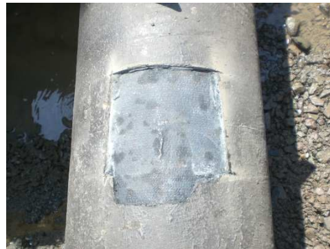
Fig. 9 Epoxy bonding layer without zinc
