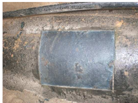
Fig. 7 Epoxy bonding layer without zinc
