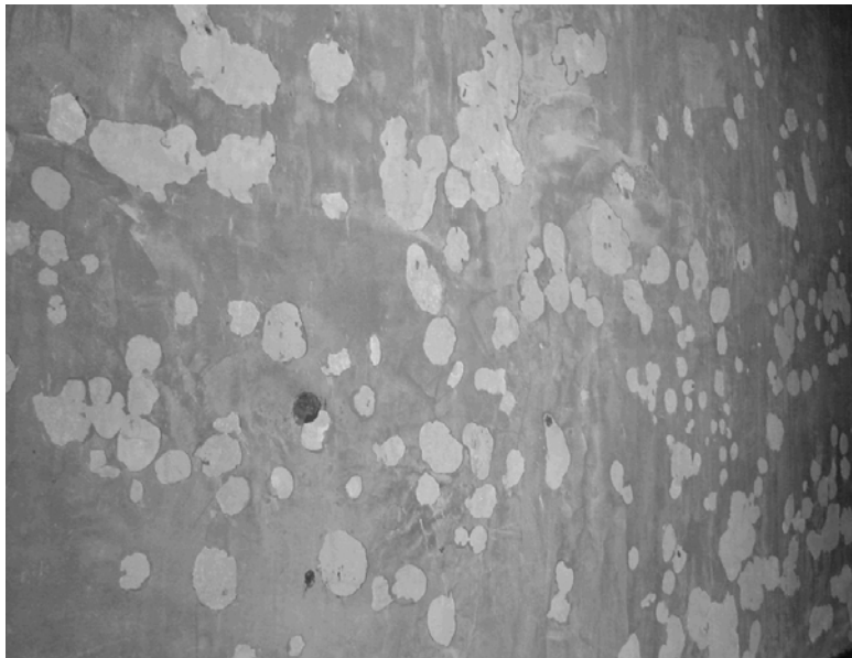
Fig. 2: Delamination on modified mortar
