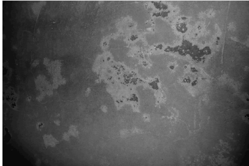
Fig. 1 different stages of alteration on cement sealing
