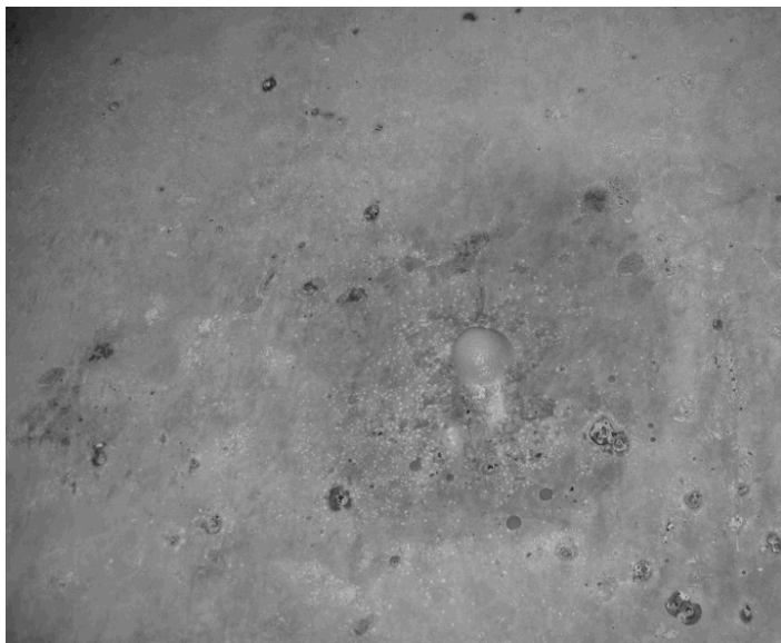
Fig. 4: Moisture and biofilm on cement sealing underlain by an adhesion layer
