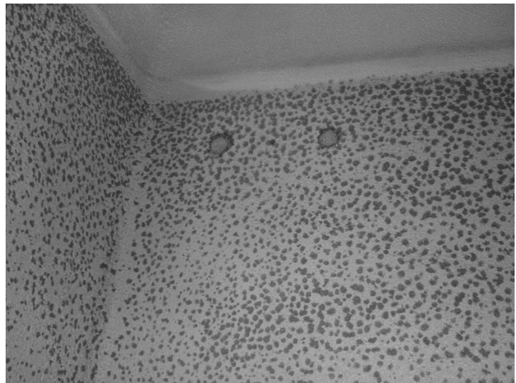
Fig. 8: Spotted alteration in tank 1
