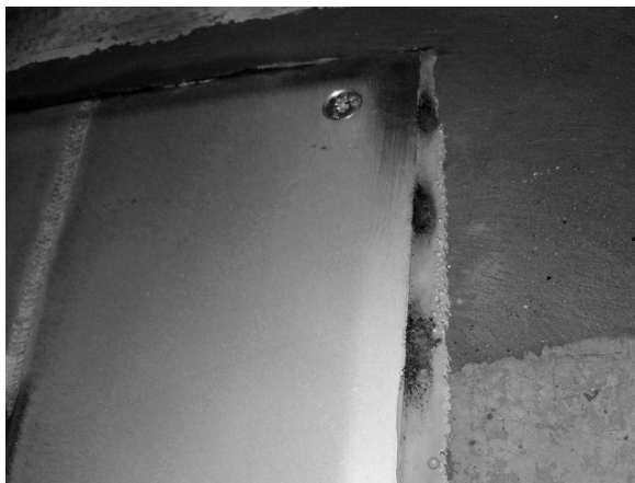
Fig. 6: Biofilm growth on door sealing
