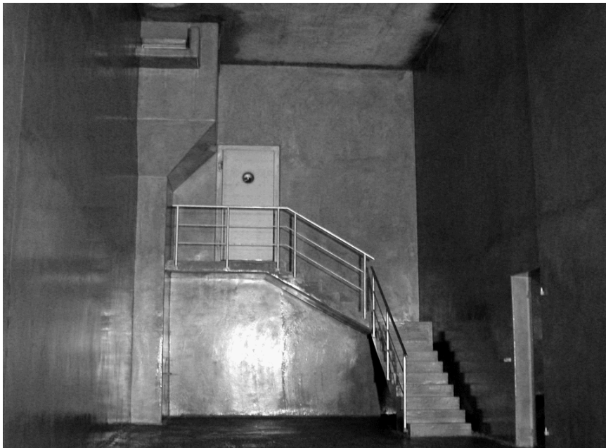
Fig. 15: Successful rehabilitation with dry process sprayed mortar, on walls, stairs, gully and over-flow
