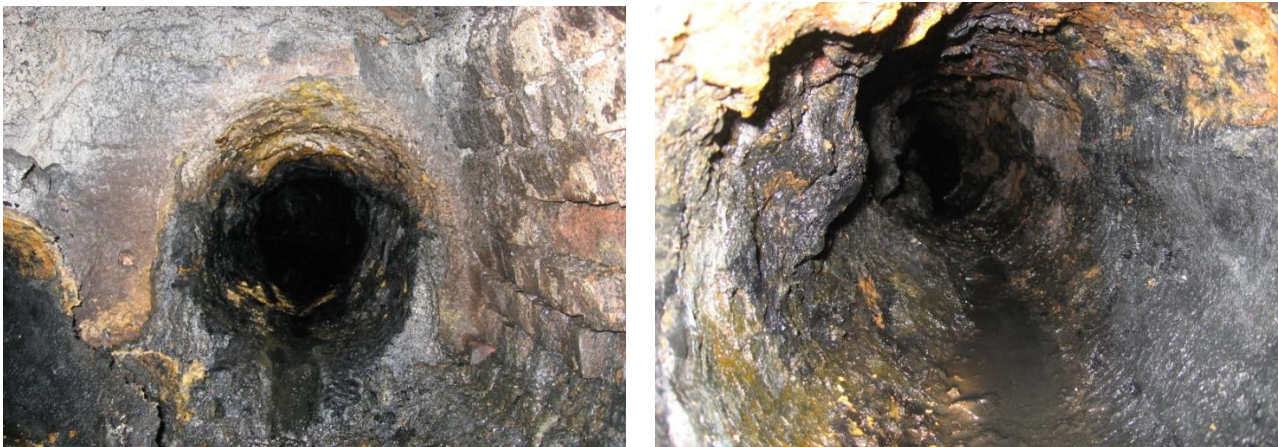
Figure 2: Illustrating the effect of hydrogen sulfide in a cast iron pressure main in Flanders (Belgium).
