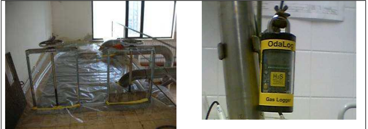
Figure 2: Adapted sewer pipe discharge point (left) and H_2S_g sensor (right)
