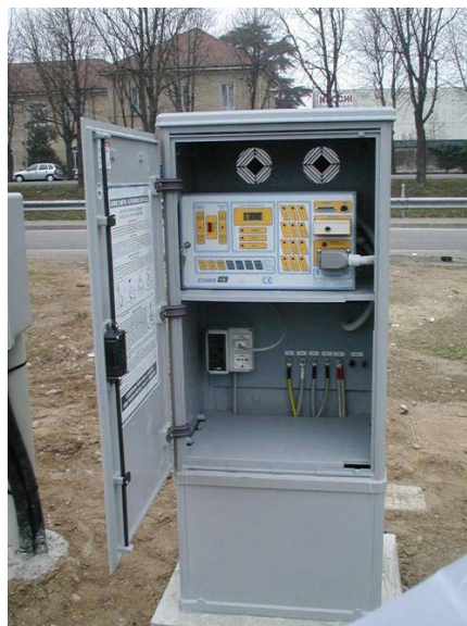
Picture 3: image of a test point with transformer rectifier
