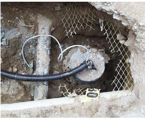
Picture 1: Examples of piping subject to corrosion with buried electrode
