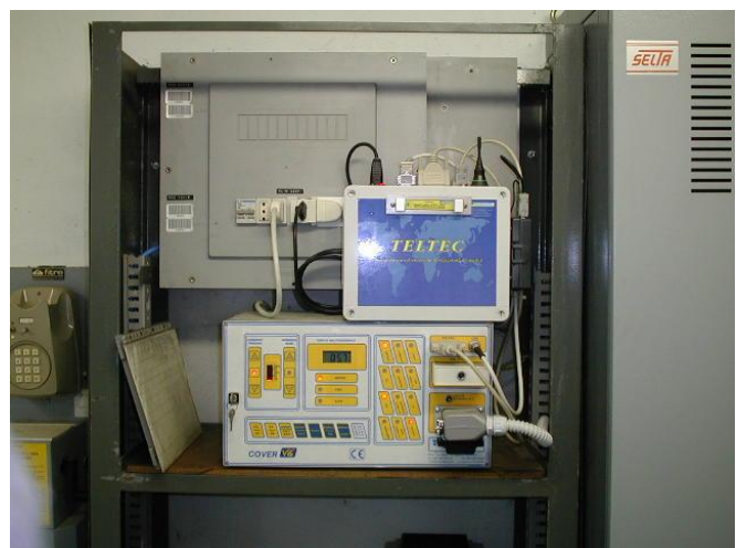
Picture 5: a test point with unit for remote control and command of the power supply
