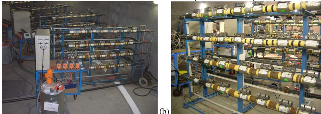
Figure 1. The whole pilot plant (a) and one of the four treatment units (b)
