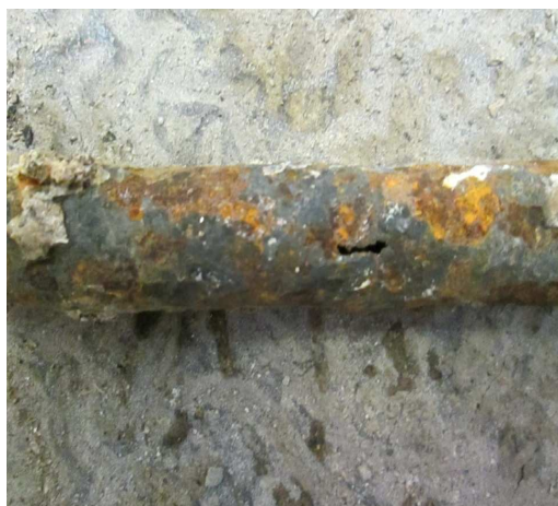
Figure 3: Damaged pipes in the kitchen area
